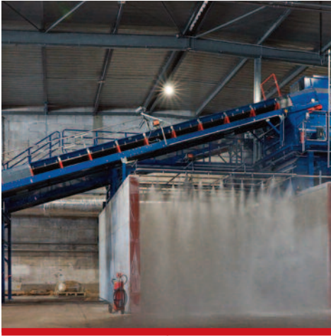
Deluge firefighting systems for enclosed areas
